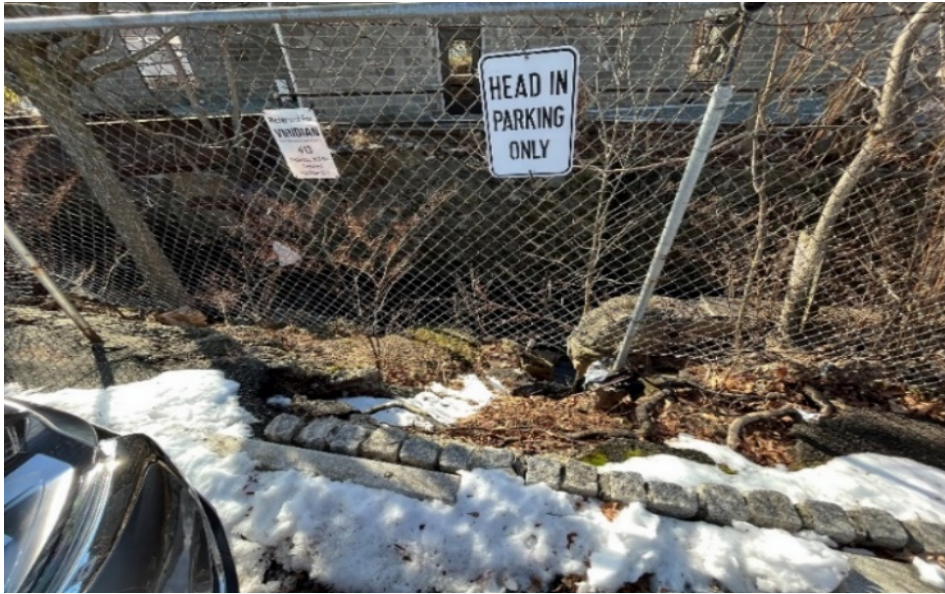
Figure 17: Visible erosion along the Second River tributary bank
